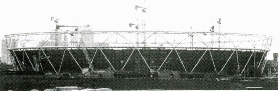
The Main Stadium, Olympic Park - 20th September, 2009 with Canary Wharf in the background. The top half of the structure is to accommodate temporary seating during the Olympic Games.
